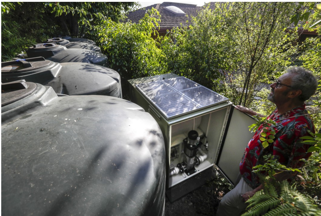
Steve Yusi installed a state-of-the-art fire-suppression system on his home located next to a wilderness area. (Robert Gauthier / Los Angeles Times)
